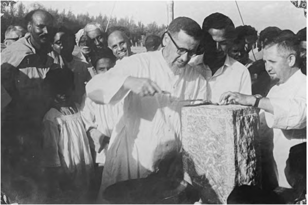
Surrounded by some Salesians and villagers, Fr. Joseph Baracca, Economer of the Province of Madras, and Fr. Emilio Dabove, Rector of Don Bosco Boys' Home, Sagayathottam, prepare the foundation-stone of Kristu Jyoti College (AKJCB).
