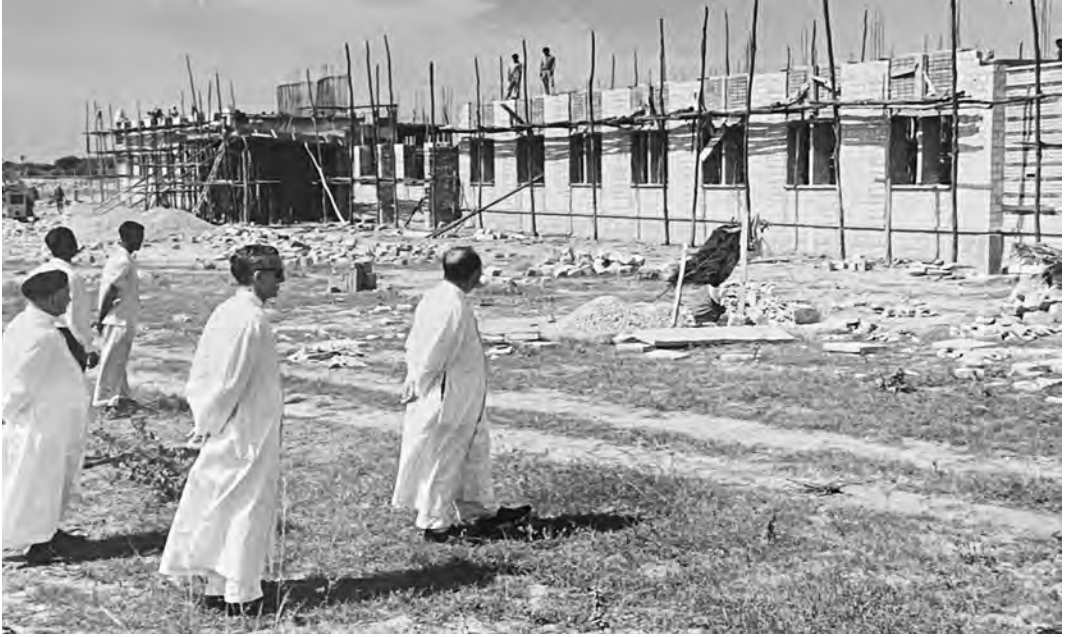
Fr. Aloysius Di Fiore, the Provincial, accompanied by two confreres, visits the construction site (AKJCB).
