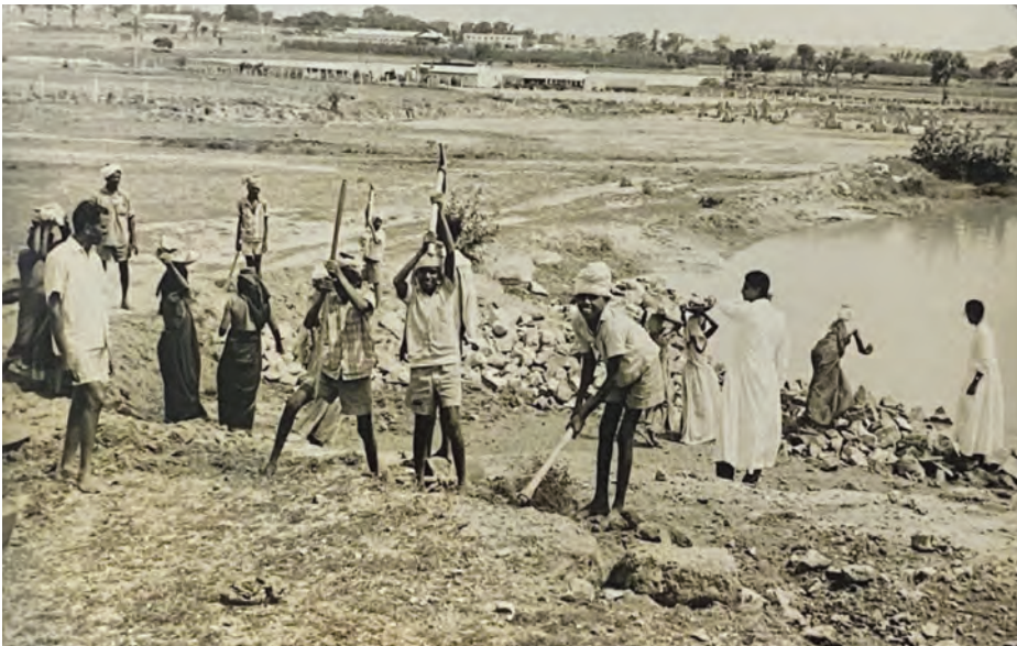
S.S.G. members with the villagers engaged in building a road to their village (AKJCB).
